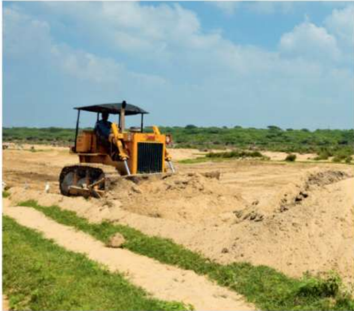
Removal of sand casting in the agricultural lands during flood caused by heavy downpour in Thoothukudi District
